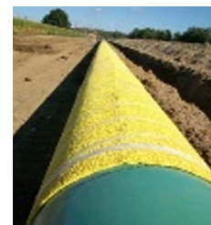
Empire Connector Interstate Pipeline Source: Tuff-N-uff
